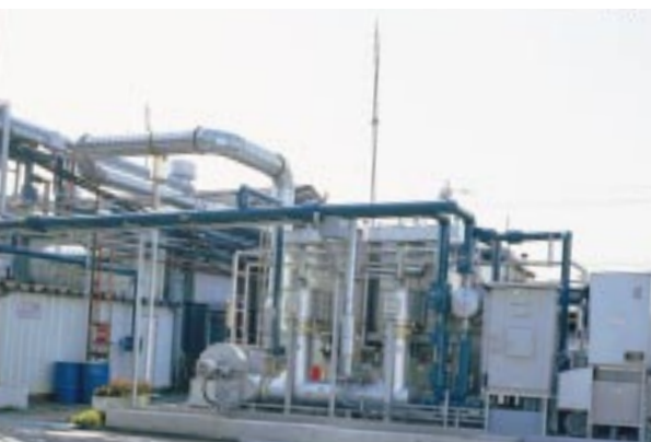
Solvent Recovery System TOHO CHEMICAL ENGINEERING & CONSTRUCTION CO., LTD.
